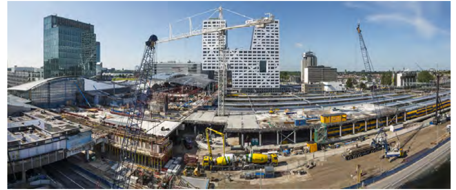
Utrecht Central station area under construction. A new and larger terminal, a new mall, the world's largest bicycle parking facility and new city hall
